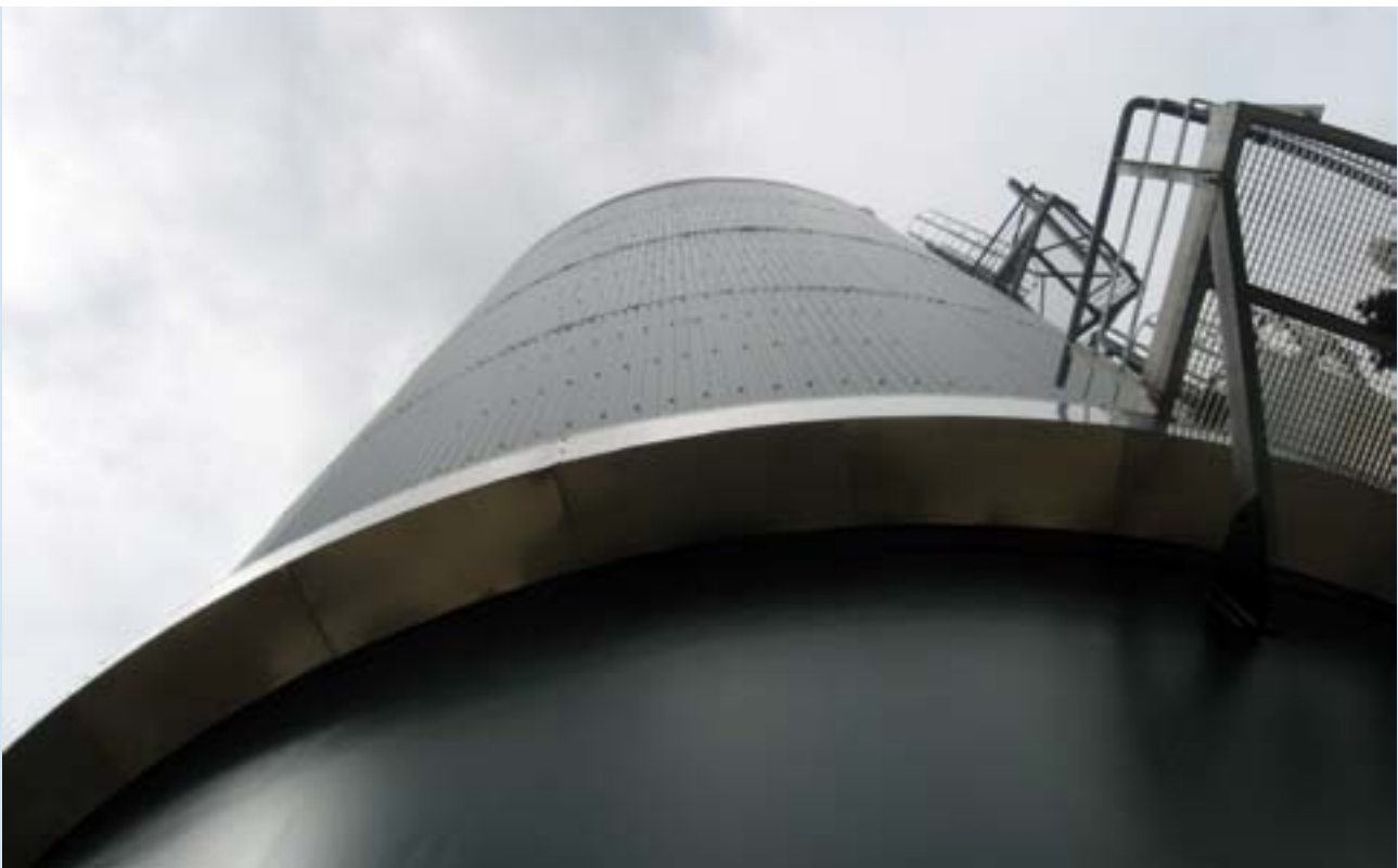
Digester of a biogas facility
