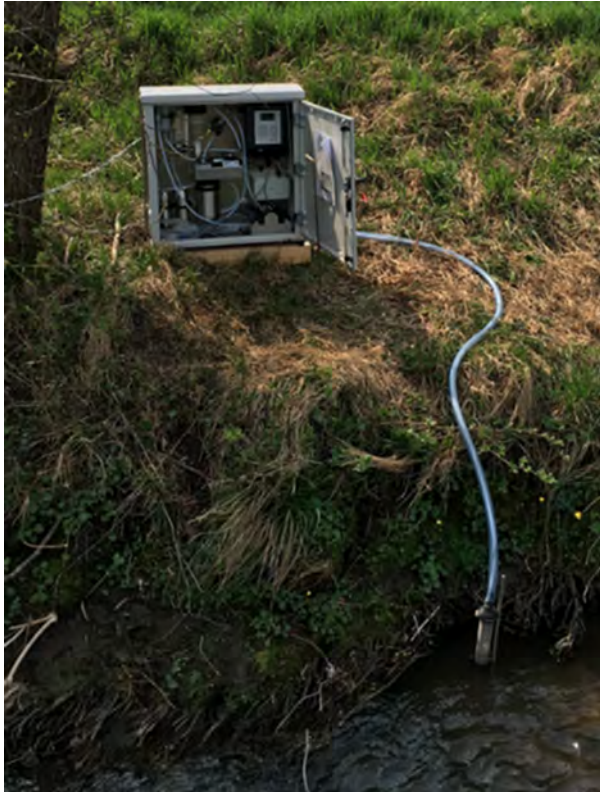
Figure 2: Automatic sampler installed at sampling site.
