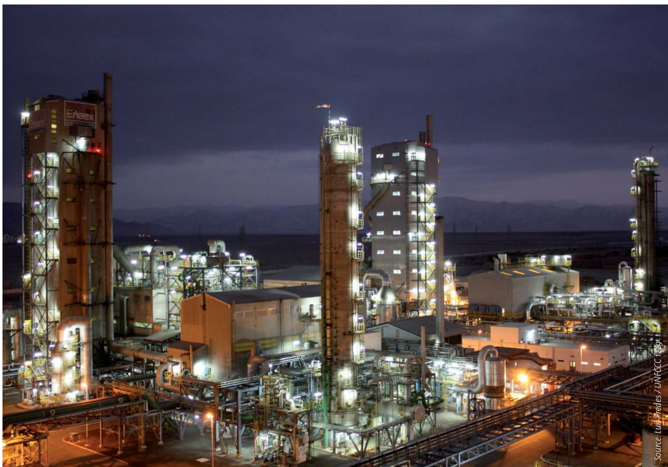
The required technology in operation: CDM project "Catalytic N 2 O Destruction Project in the Tail Gas of the Nitric Acid Plant PANNA 3 of Enaex S.A."
